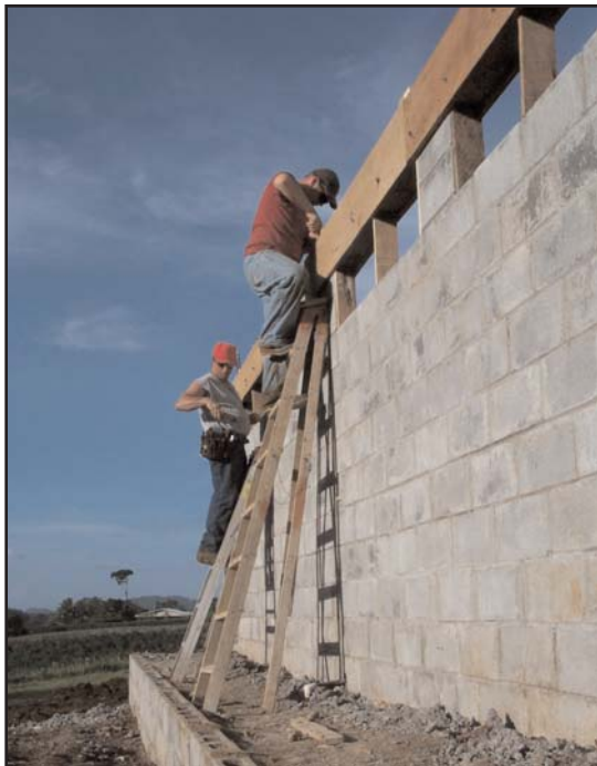
Tim Fields & Jeremy Yancey from Bethel Life Center in Wichita, KS, prepare forms for the bond beams.
