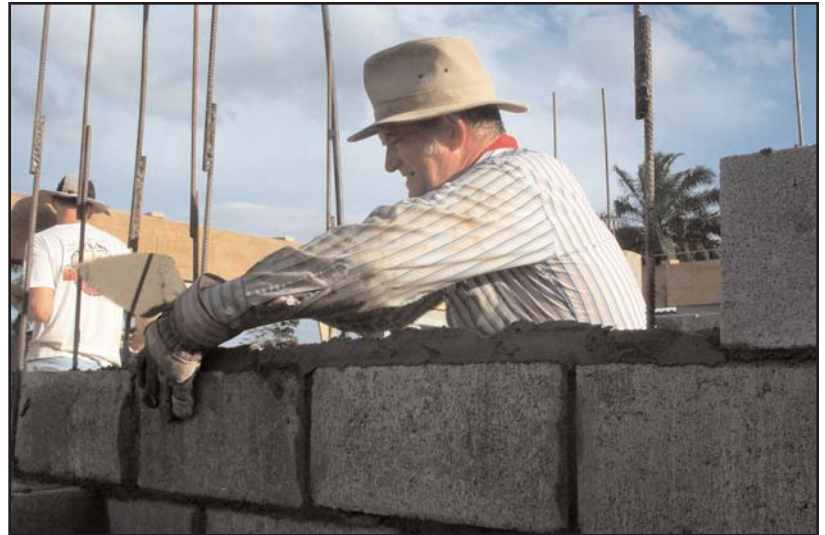
Terry Haslinger from Bethel Life Center in Wichita, KS, lays block on a cabin.
